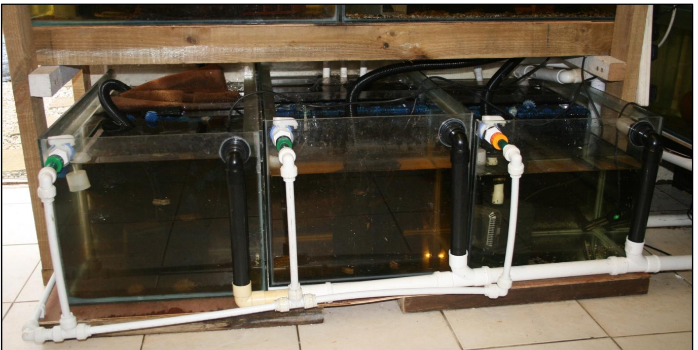
Separate sumps for each of three centralised systems. Photo: M. Walters
