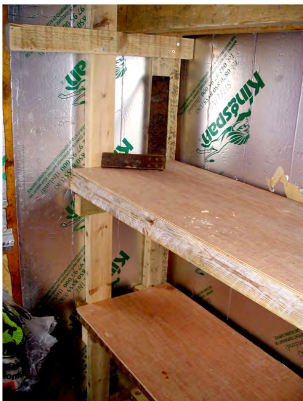
Shelves constructed with a plywood tank base
